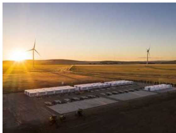
South Australia's huge battery storage project is being expanded – Hornsdale Power Reserve
