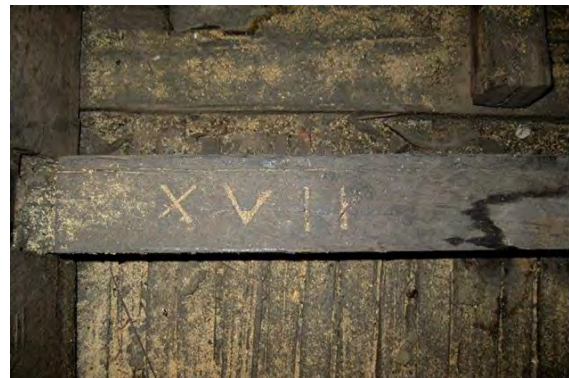
Timbers in The Mint were probably sawn from timber cut in Lane Cove during 1812 and 1813; the ceiling joists are all numbered in Roman numerals (photo Ralph Hawkins)
